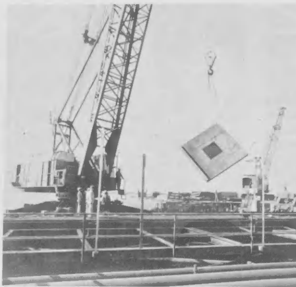
One of the two-ton concrete slabs is carefully lifted from the walkway to permit work on the steel structure. Uno di e planchanan di concreet di dos ton ta ser hiza cu cuidao aki pa permiti trabao ariba e estructura.
